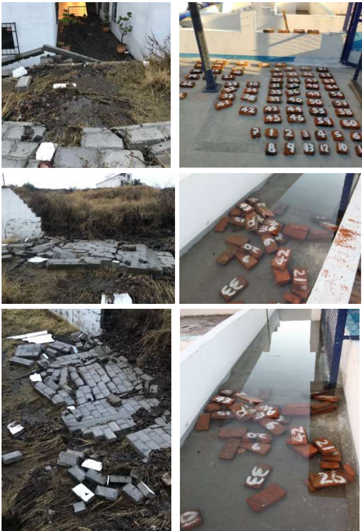
Figure 7 Failure of the brick wall during the storm 13-14 June 2018 and successful reconstruction of wall failure in forensic analysis channel.
